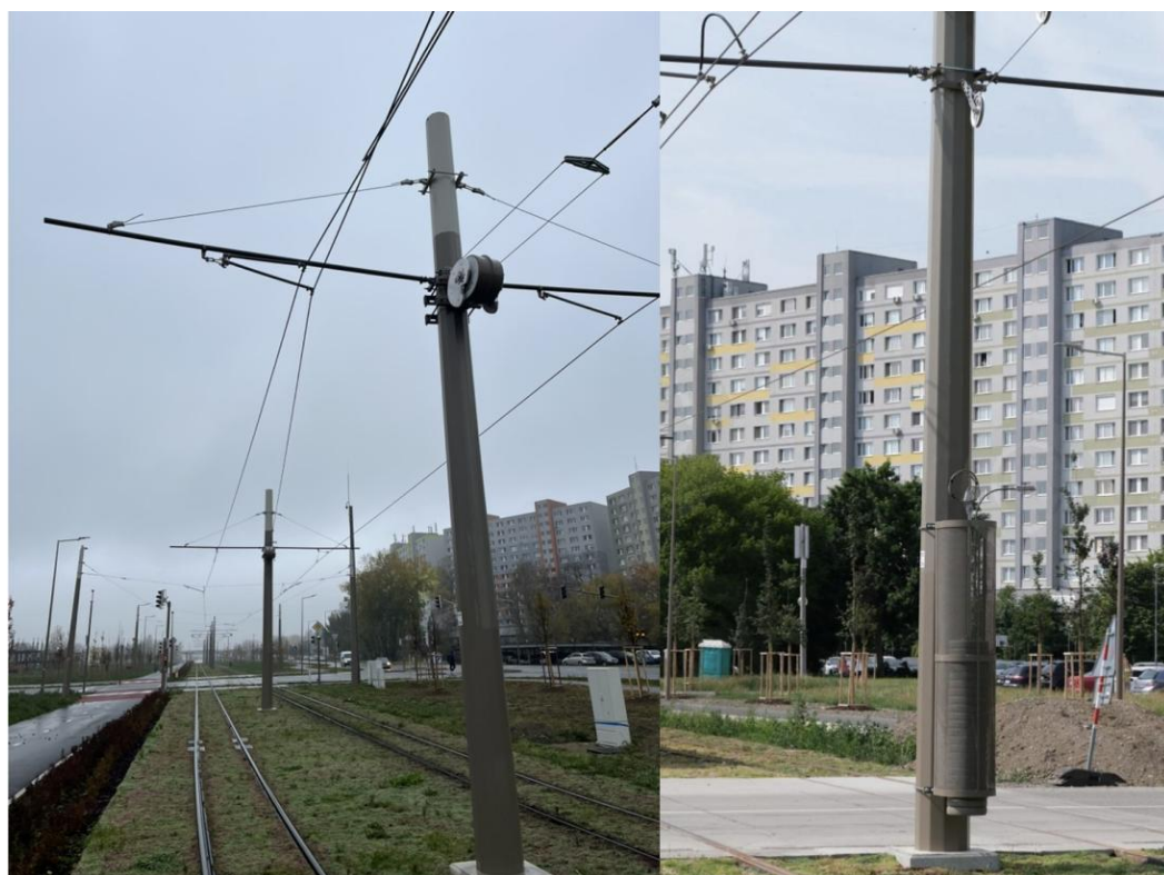
Figure 10. Two methods of tensioning the overhead contact line. On the left, using a tension pulley, on the right, using the addition or removal of weights. In the figure on the left, we can also see the ongoing replacement of overhead contact lines within the exchange field. Source: Own photograph.
