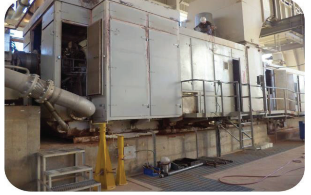
Fig. 1. GE MS 5001P Gas Turbine
