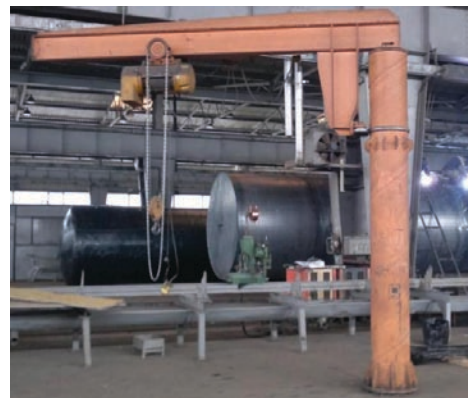
Fig.1. Console crane in working environment
